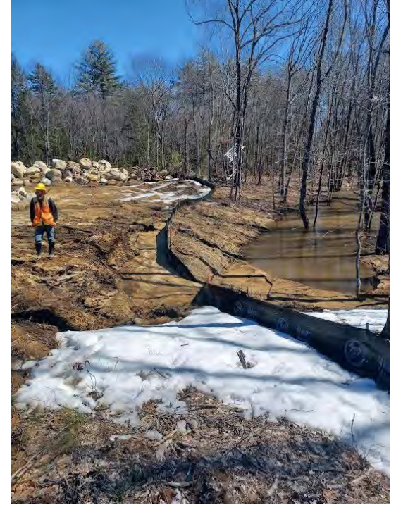
Silt fence over-topped
