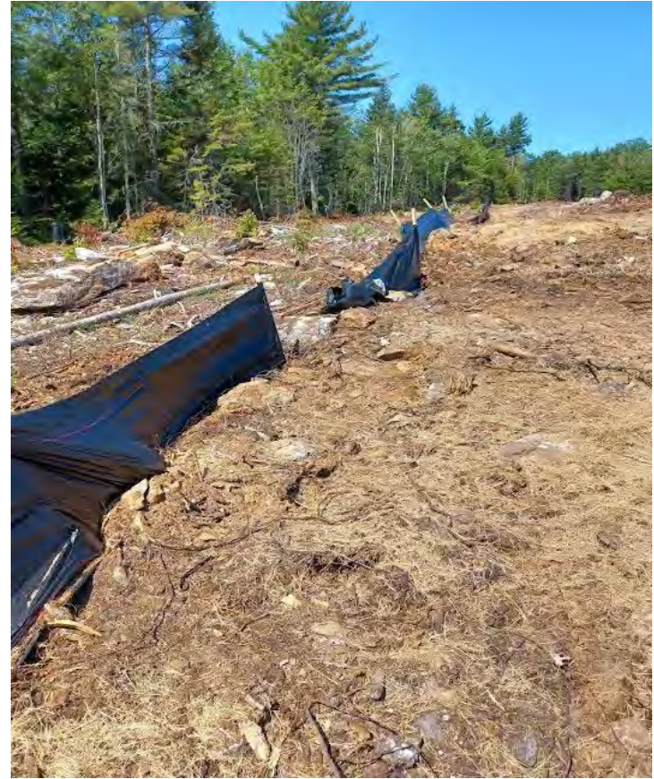
Silt fence not continuous, and not keyed in
