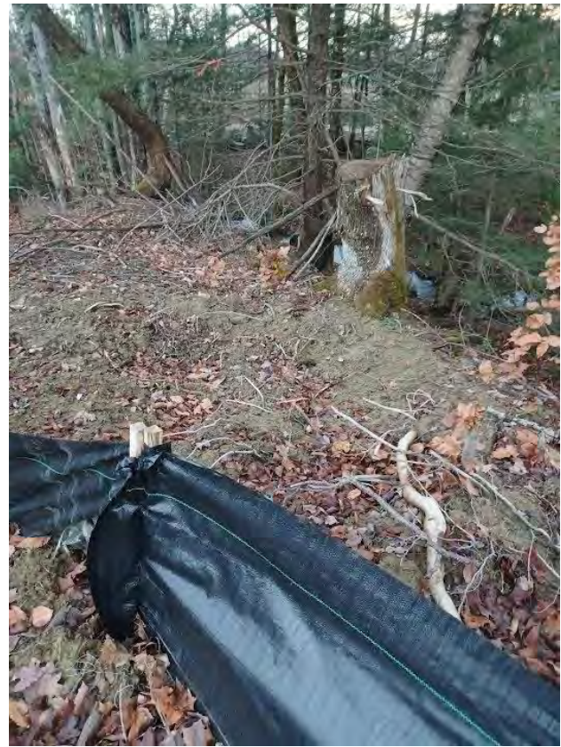
Silt Fence not sited at edge of disturbance, and not keyed in, discharging to unnamed stream
