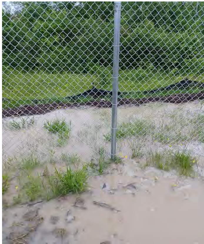
Silt Fence overwhelmed and not maintained, discharging to unnamed stream
