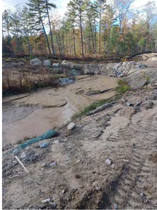
Sediment basin at capacity and no longer functioning
