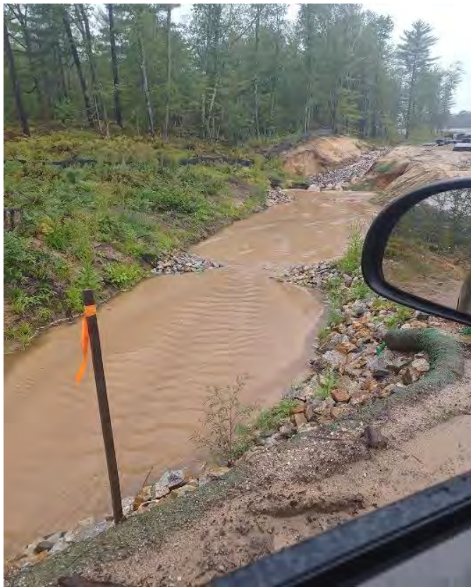
Failing sediment basin discharging to unnamed stream
