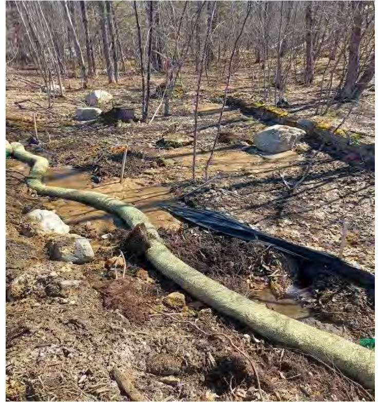
Straw Wattle, overwhelmed and not anchored
