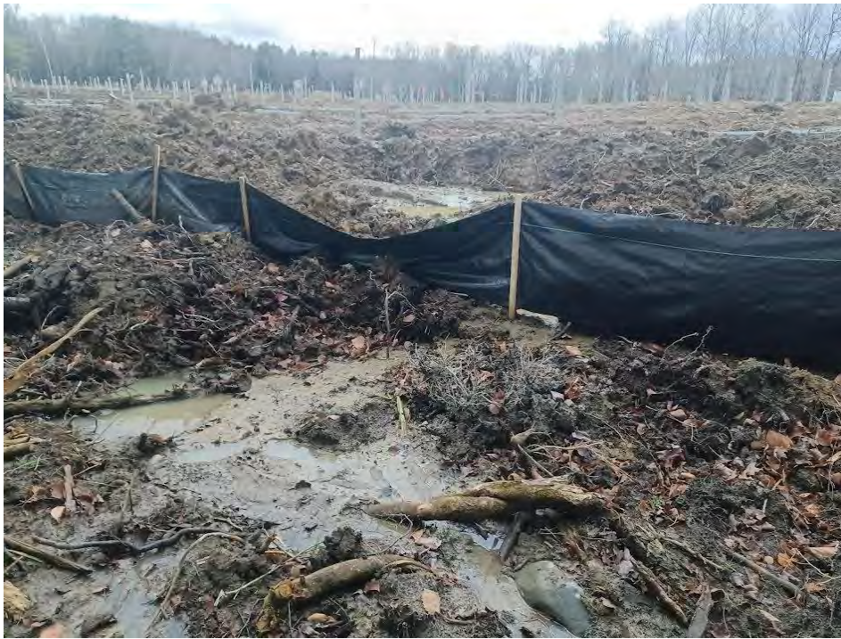
Silt fence not keyed, placed in drainage swale discharging to wetland of special significance and unnamed stream
