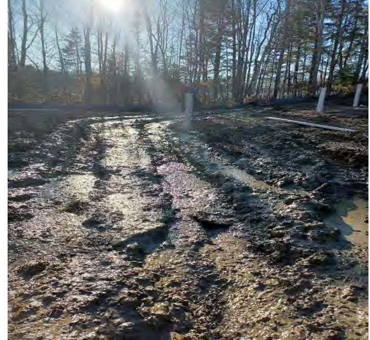
Solar Project causing wetland discharge (left); Solar project causing stream discharge (right)
