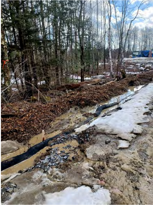
Silt sock not installed on contour and directing flow to unnamed stream
